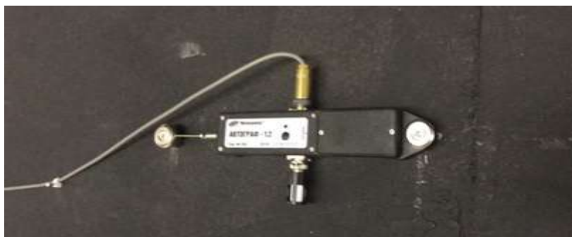
Figure 7. – Electronic beacons – registrars «Autograph – 1,2» placed on the crack of the beam beam (main) BPN – 3.13, section in the B, 6 – 7 axes
