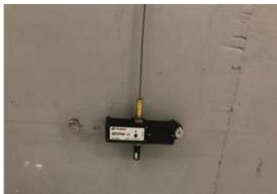
Figure 6. – Electronic beacons – registrars "Autograph – 1,2" placed on the crack of the beam beam (main) BPN – 8.13, section in the K, 11 – 12 axes
